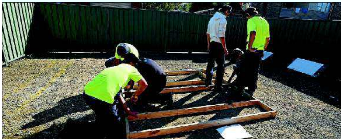
Framework is pieced together at the ATEL Wagga Wagga Pre-Apprenticeship Carpentry/Construction Course. Pictures: Addison Hamilton
